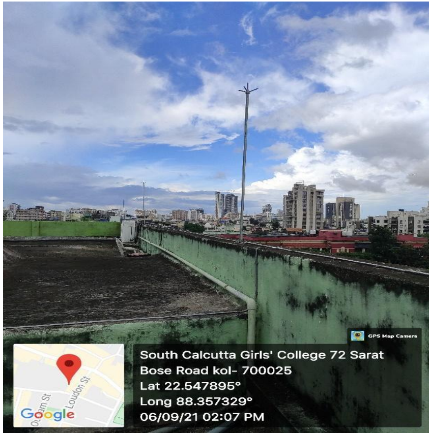
LIGHTNING ARRESTER ON ROOFTOP
