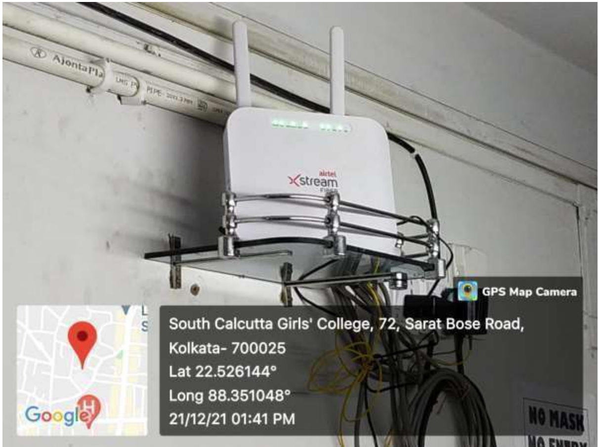
NEWLY INSTALLED Wi-Fi ROUTER FROM AIRTEL
