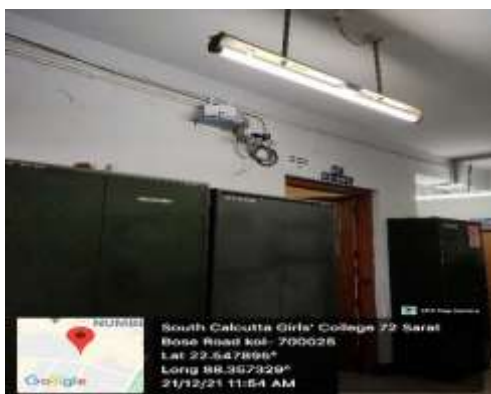
INTERNET FACILITIES ARE EXTENDED WITH ROUTERS IN EACH FLOOR
